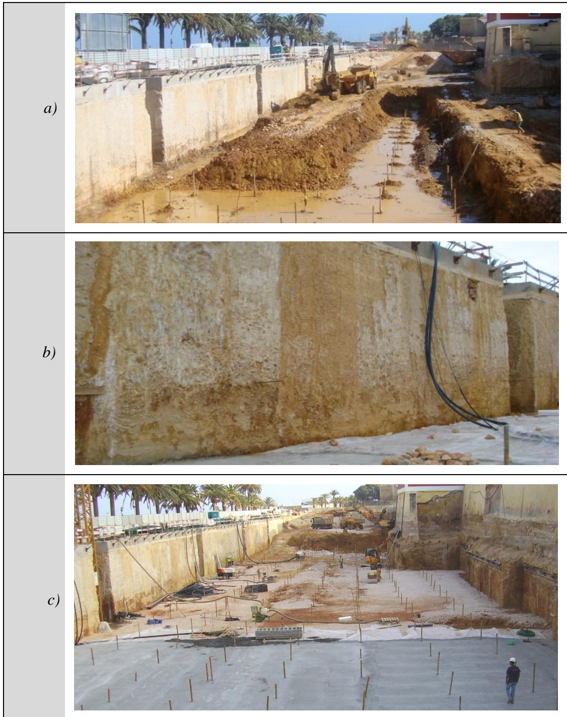
Figure 9: Views of the work during the excavation: a) excavation of 6 m depth; b) detail of the CSM wall; c) regularization of the bottom of the excavation.
