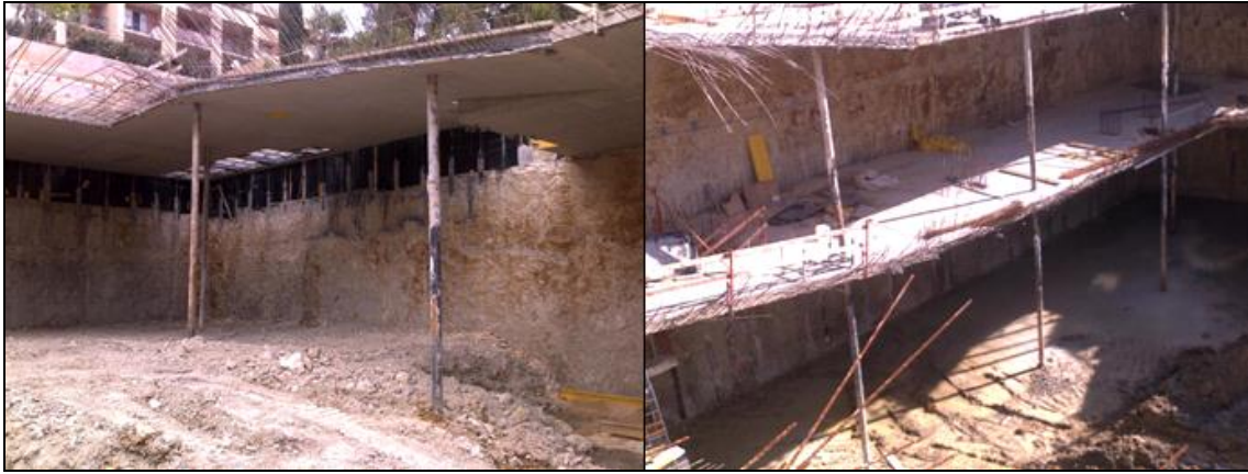
Figure 11: View of the work during the second level of excavation (on the left) and after the execution of the second level of slab bands (on the right).
