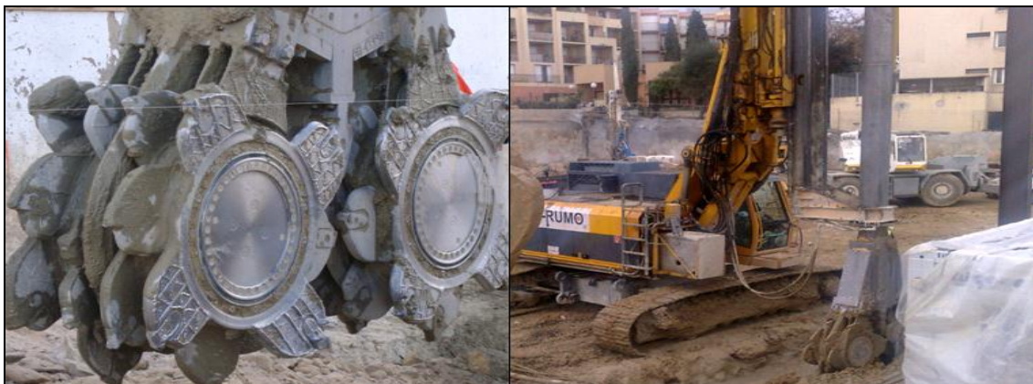
Figure 3: Detail of the cutting wheels (on the left) and general aspect of the hydromill (on the right).
